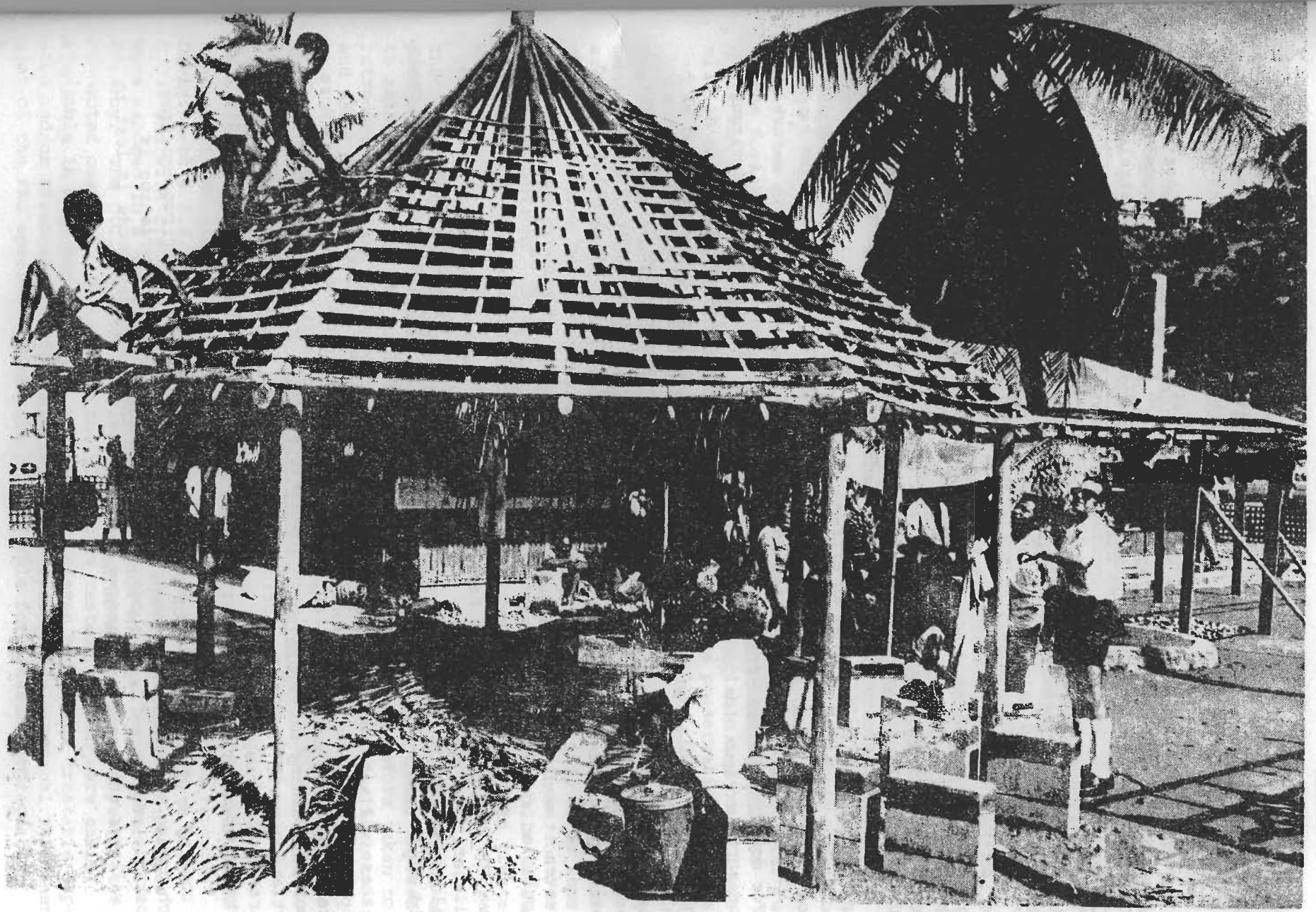
A simple market stall using treated Teak and Bamboo in Port Moresby.
