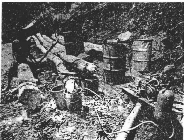
Treating logs by H.P.S.D. using a 12.5cm cap. Pump and manifold can be seen in foreground.
