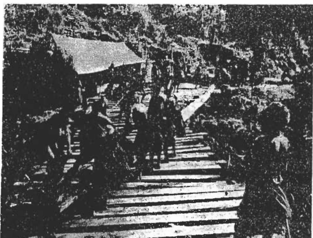
Hauling a 12m Casuarina oligodon log over the old bridge for H.P.S.D. treatment.
